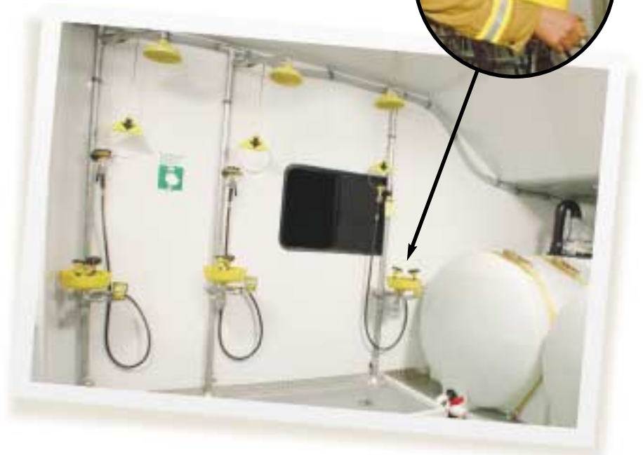
Decontamination Showers and Water System
